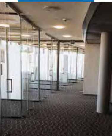
Montaj mocheta in Centul Postal utilizand Ultrabond Eco Fix - Post Tower - Italia
