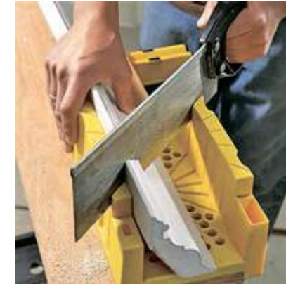
Cut the cornice using a saw and a mitre box. Use a 45-degree angle for standard corners.
