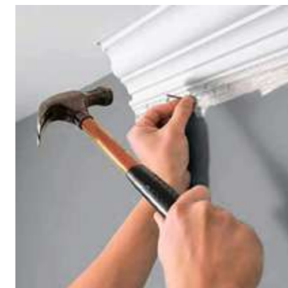
Secure the cornice with finishing nails to prevent sliding while the adhesive sets. Ensure joints are perfectly aligned.
