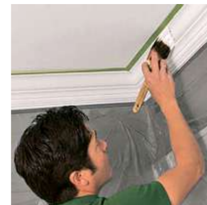
Protect walls and ceilings with masking tape. Paint the cornice using a brush or spray (do not use acetone-based paints).
